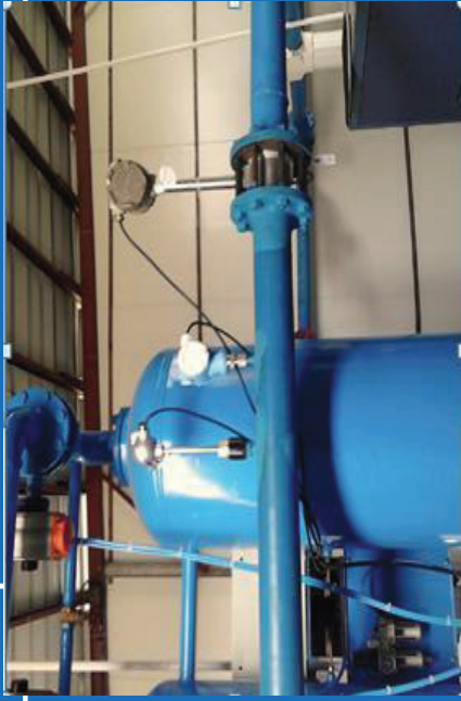
Compressed Air Measurement On Site
