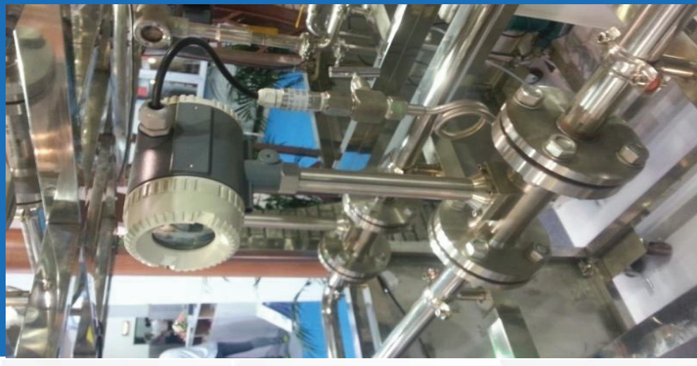
Steam Measurement On Site
