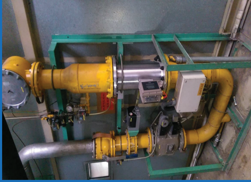
Coal Gas Measurement On Site
