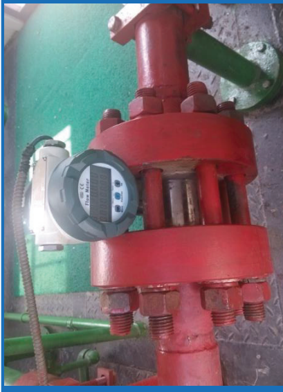
On Diesel Measurement
